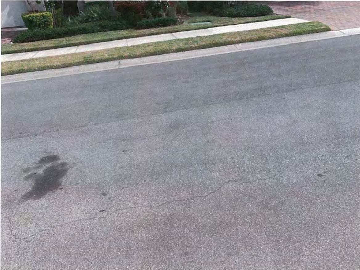
Photo suspected reflective cracking Ventosa Place
