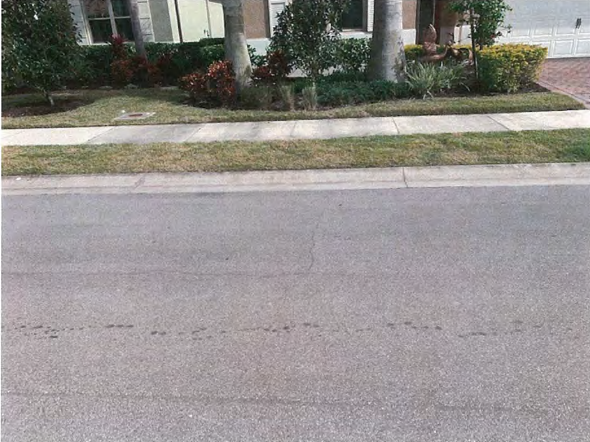
Photo of suspected reflective cracking Ventosa Place
