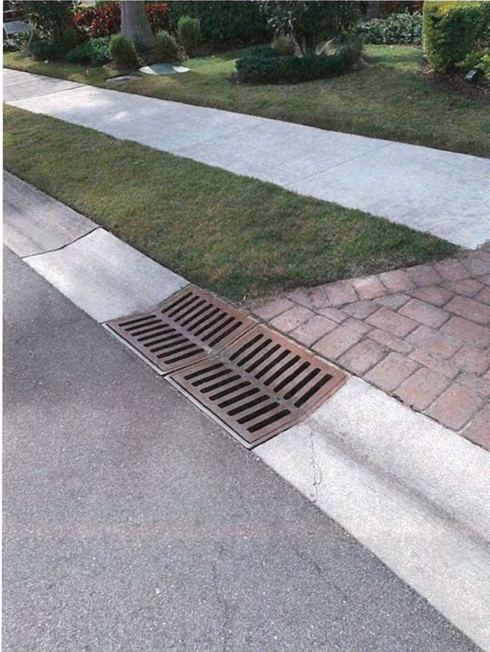
Photo stress cracking Ventosa Place
